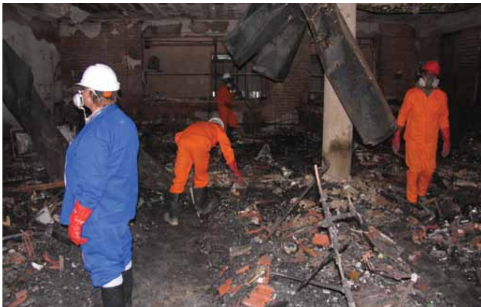
FACTORY POST FIRE CLEAN-UP
